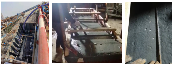
图8 钢混结合段预应力张拉端密封部位 Fig. 8 Sealing part of prestressed tensioning end of steel-concrete joint section Fig. 9 UHPC pouring
